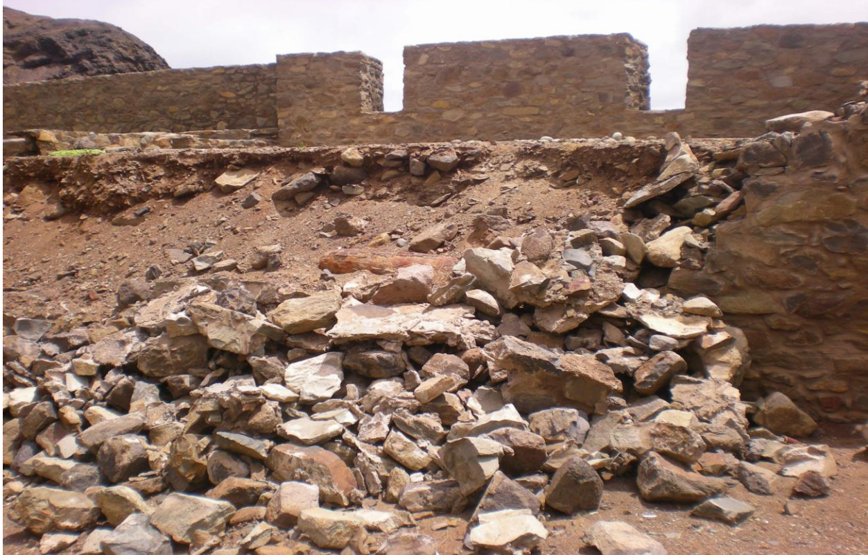
Figure XX - Collapsed portion of newly repaired wall, Sandy Bay Lines
